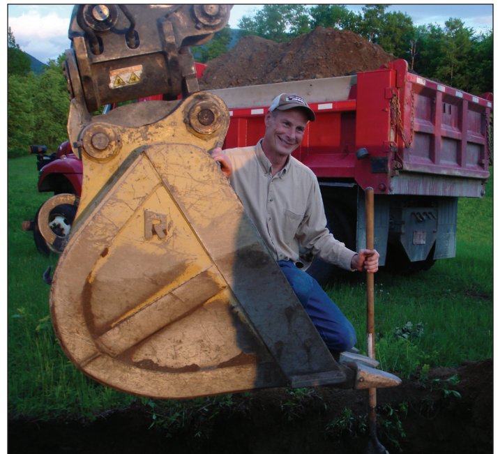
Kurt Johnson is lowered via excavator bucket into a 9 foot hole, so he can square off the corners and edges in order to fit the time capsule.
