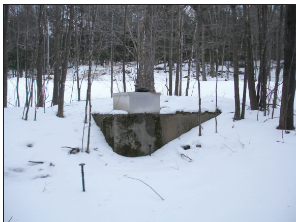
Figure 5. Maple Ridge Cistern
